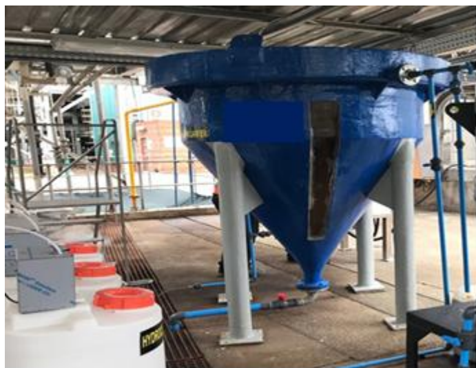
Fig. 1 Clarifier set up
