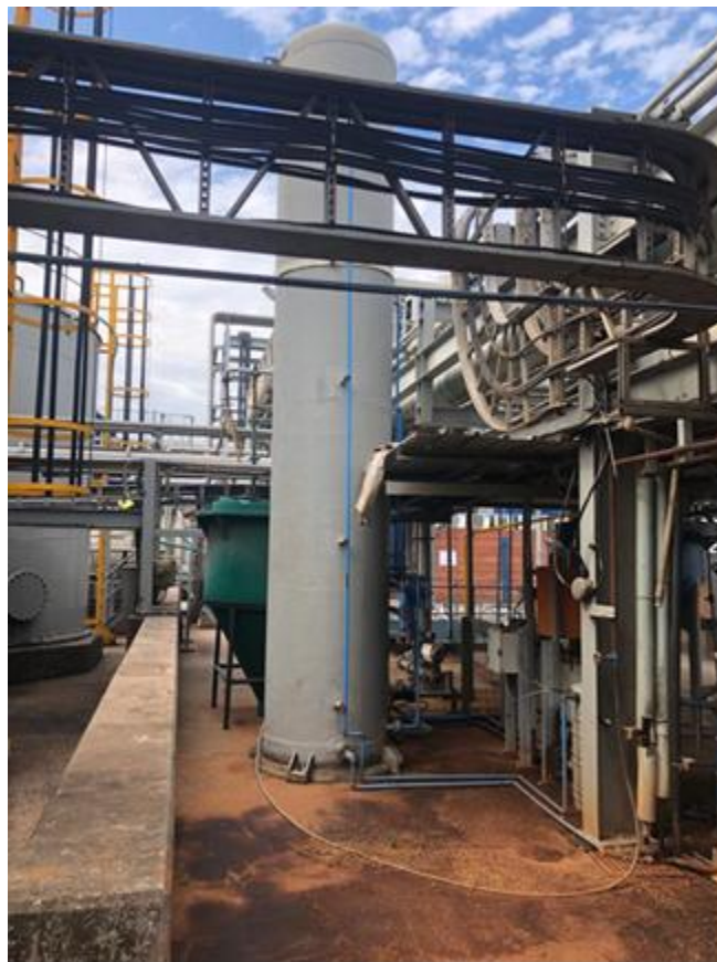
Fig. 2 Anaerobic Digester set up
