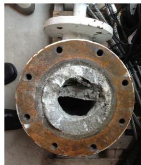
Fig. 1 Struvite formed in pipeline
